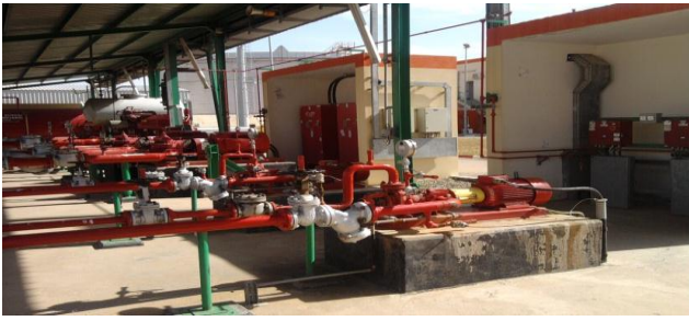
Figure (2.10) : Central anti-incendie.
