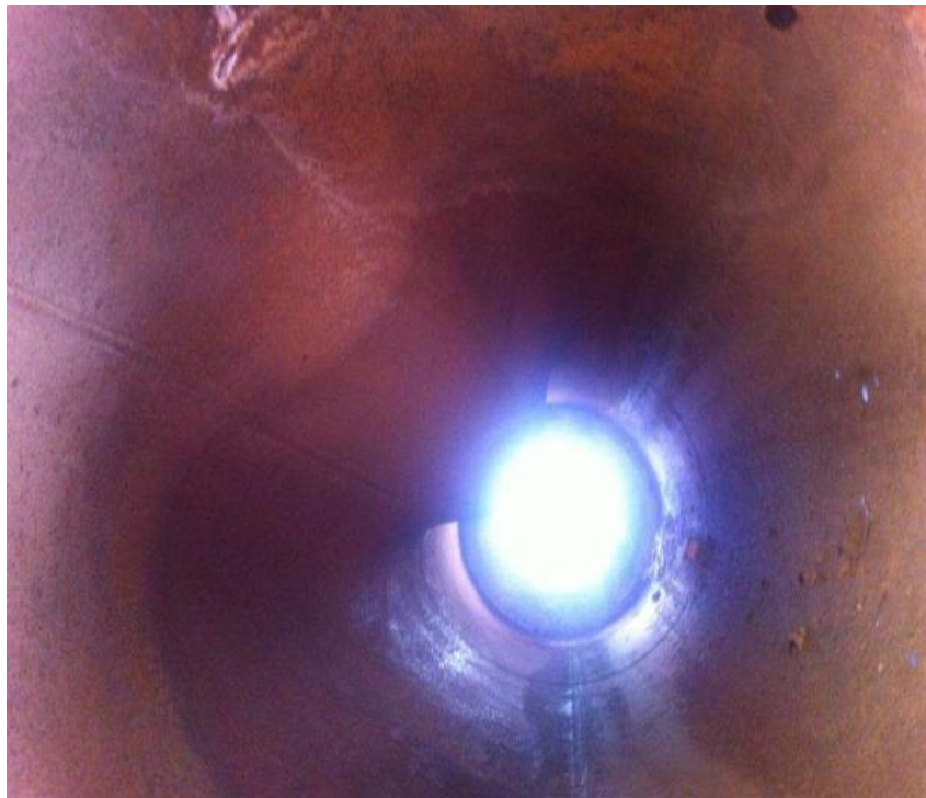
Figure IV.14. Hernia formed on an old German boiler of the customer [1].
