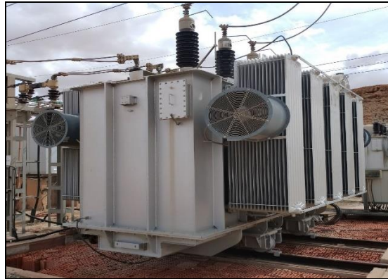
Figure.III.2: post 60/30 KV a Bousaâda.
