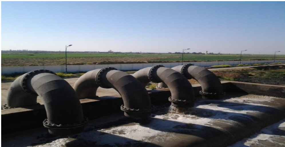
Figure II.4 : post de relevage
