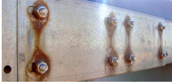
Fig I. 3 Galvanized mild steel cable ladder with corrosion around stainless steel bolts
