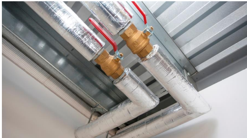
Figure 15: tuyauterie de chauffage
