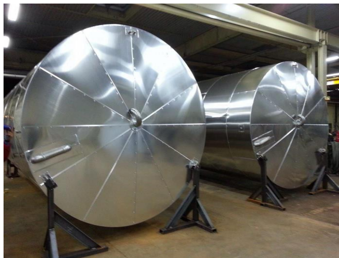
Figure 14: cuve de stockage
